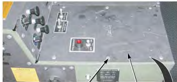
SCREWS CIRCUIT BREAKER NO. 11 LEFT HEATER COVER
