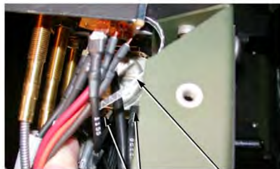
TEMPERATURE CONTROL SWITCH TERMINALS
