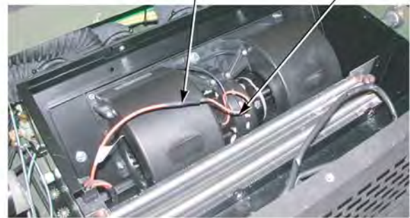
AC HEATER/EVAPORATOR BLOWER MOTOR GROUND WIRE AC HEATER/EVAPORATOR BLOWER MOTOR CASE
