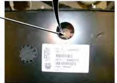
AC CONDENSER DRYER SIGHT GLASS
