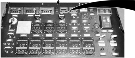
PUMP OPERATOR'S PANEL
