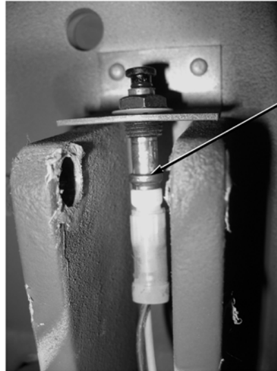
EQUIPMENT (LADDER) RACK LIMIT SWITCH
