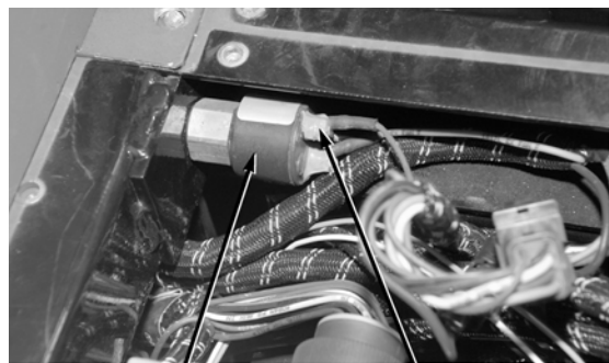
PUMP HOUSE COOLING FAN TEMPERATURE SWITCH
