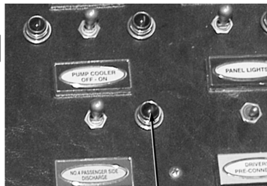
PUMP COOLER INDICATOR
