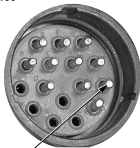
TERMINAL J WIRE 1188
