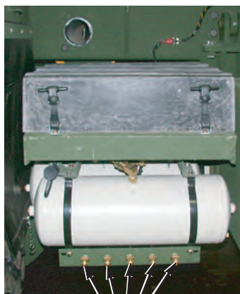
AIR RESERVOIR DRAIN VALVES
