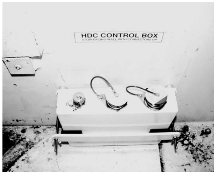
Figure 5-19. HDC Control Box
