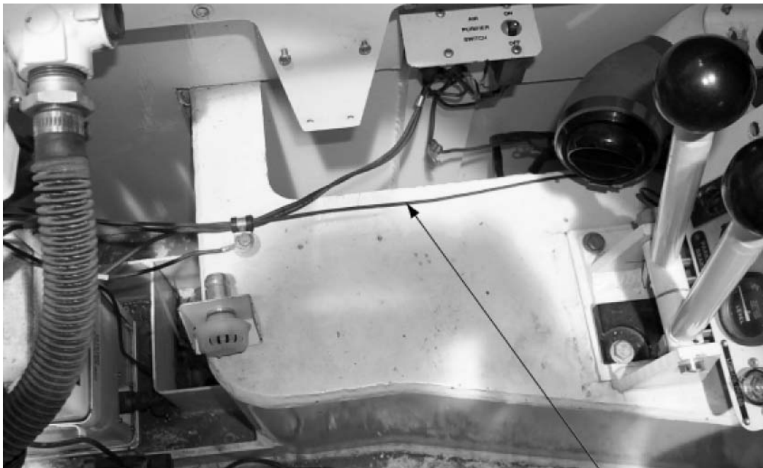
CABLE ASSEMBLY W1 BRANCH 1069 FROM DISCONNECT BRACKET
