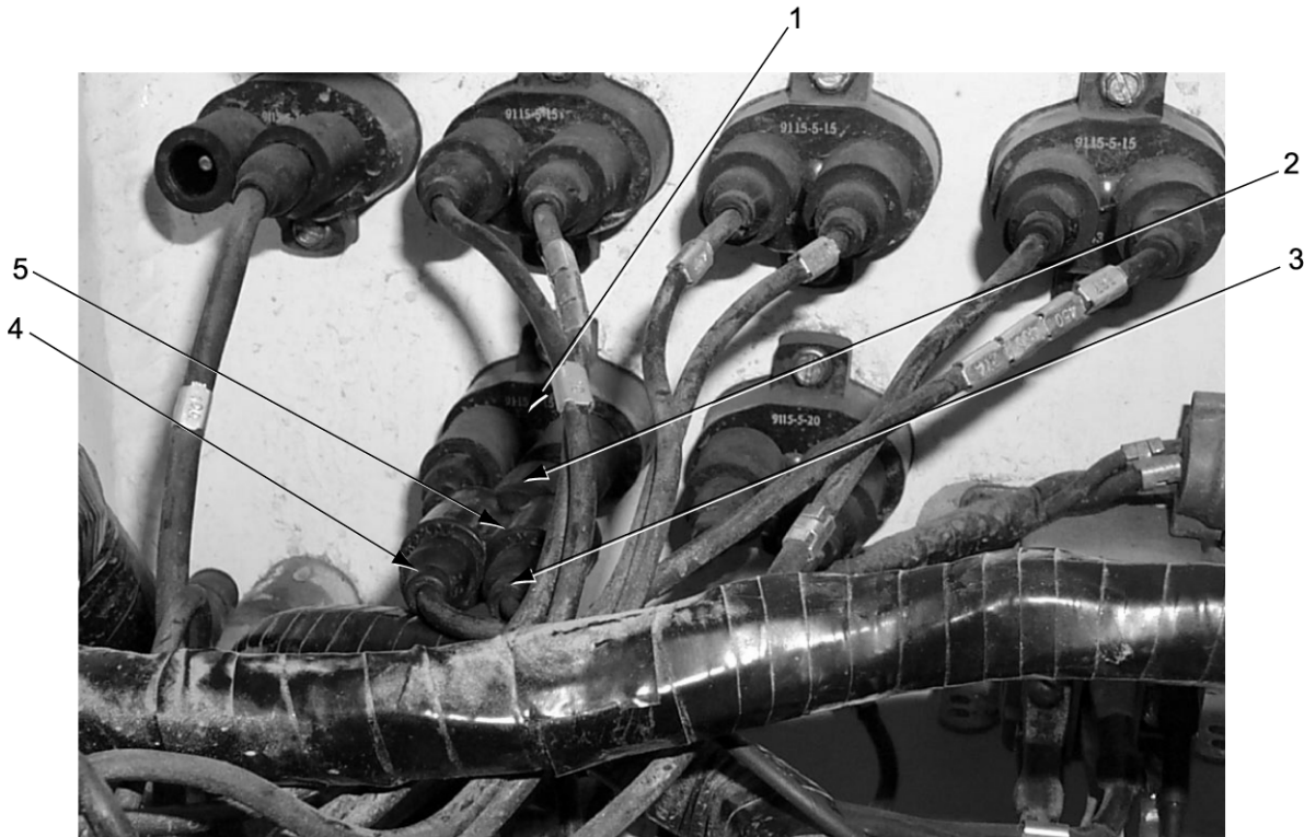
Figure 5-7. Connection of HDC Power Distribution Components
