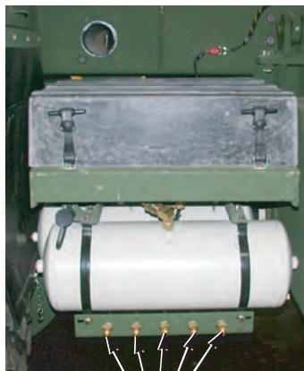
AIR RESERVOIR DRAIN VALVES
